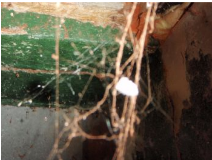
Rotting Window Header
