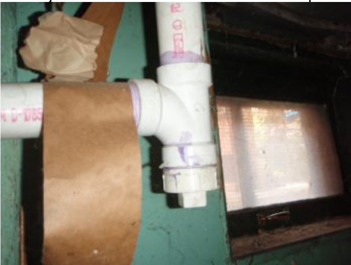
Improperly Installed Cleanout is Highly Vulnerable to Clogs
