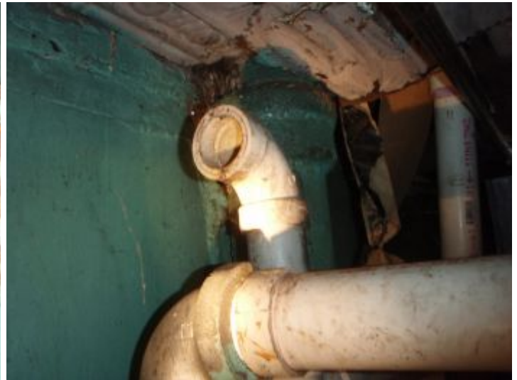
Open Waste Pipe in Basement
