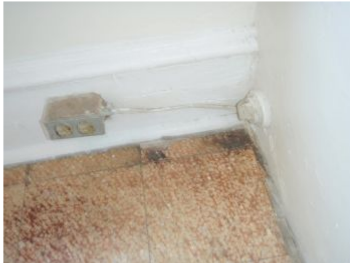
Exposed Wire Run in Kitchen
