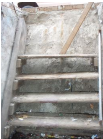
Damaged Stairs to Basement
