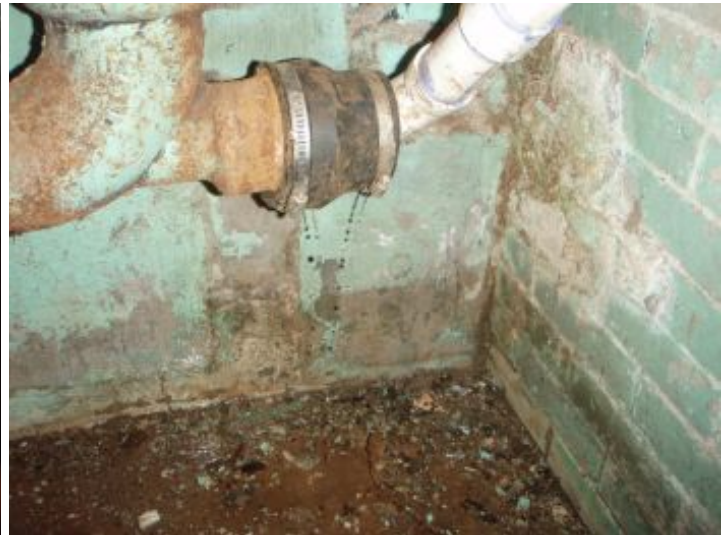
Leak at Drain in Rear Section of Basement
