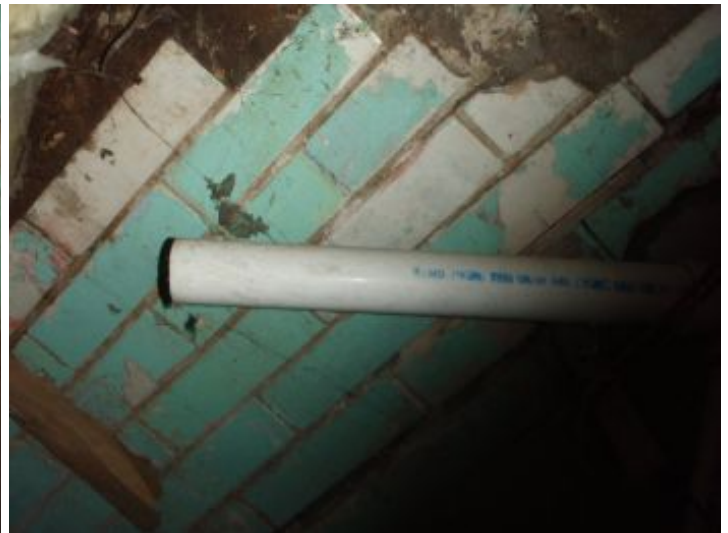
Open Waste Pipe in Basement
