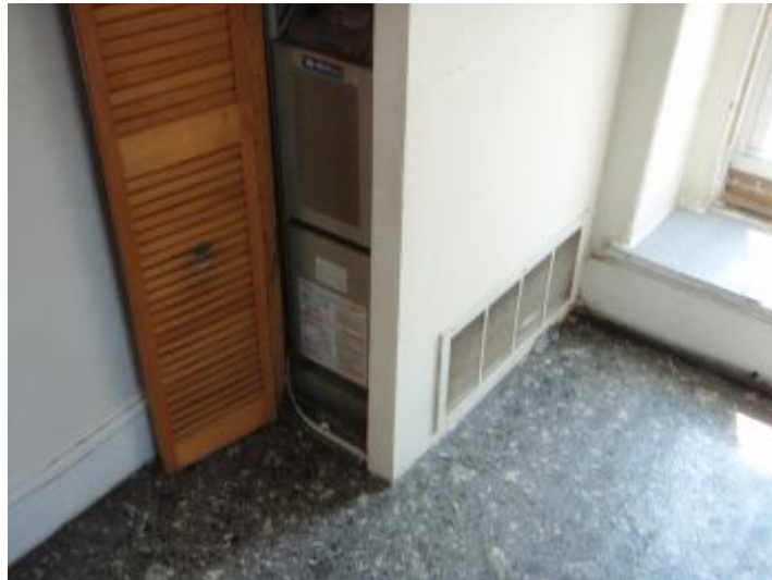
Combustion and Return Air Sources are too Close and Can Mix
