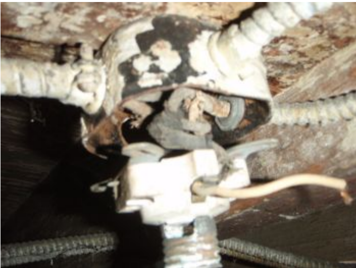
Exposed Wires at Light Fixture in Basement
