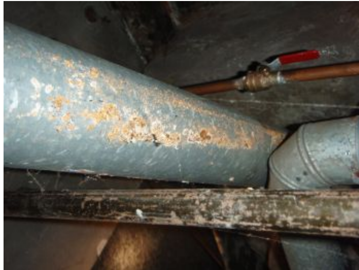
Corrosion Noted on Underside of Vent Pipe Indicating Possible Drafting Problems
