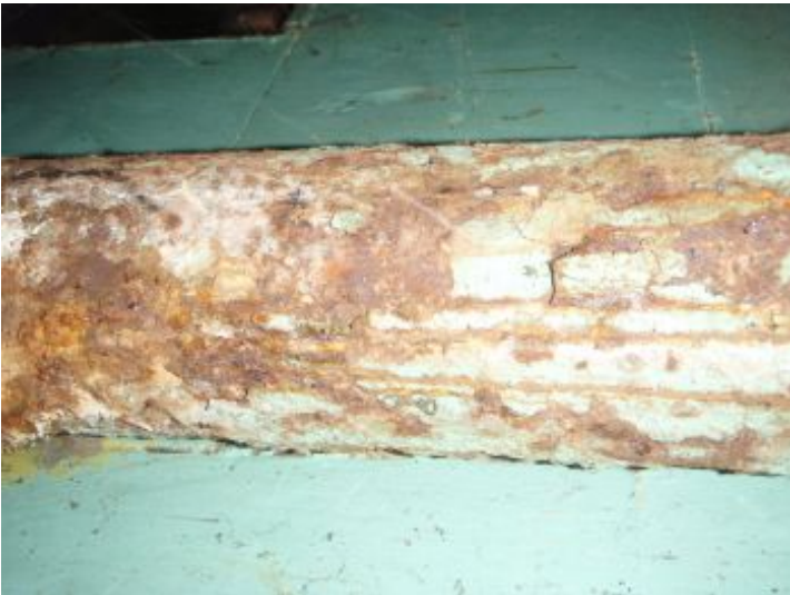
Major Corrosion Noted at Cast Waste Pipe
