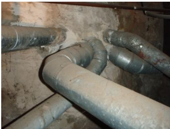
Six Gas Appliances Vent to the Same Chimney Flue
