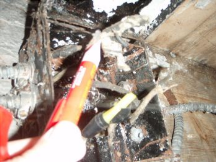
Exposed Wires Noted in Basement
