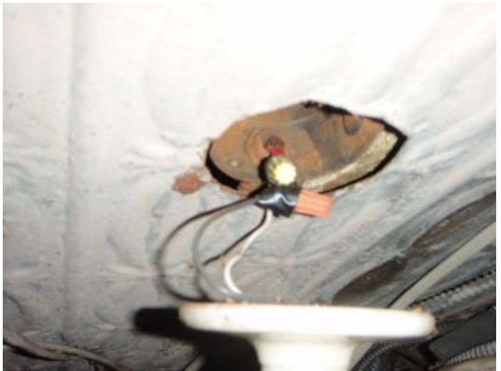
Exposed Wires at Light Fixture in Basement
