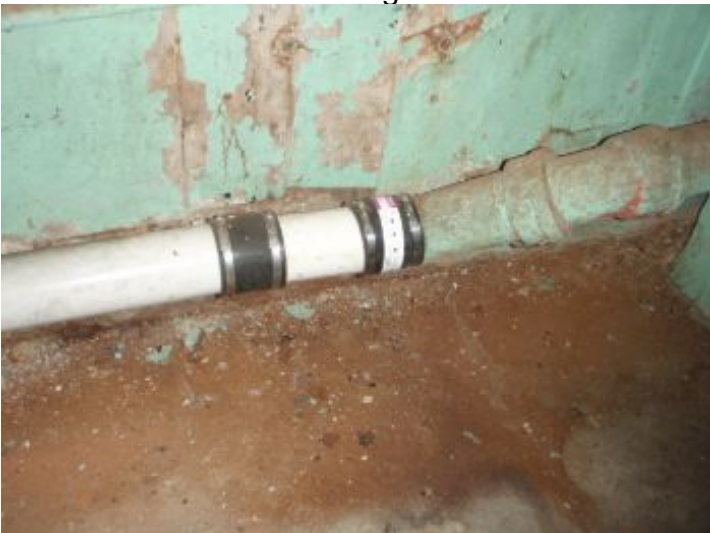
Missing Shear Rings/Waste Pipe Not Properly Supported
