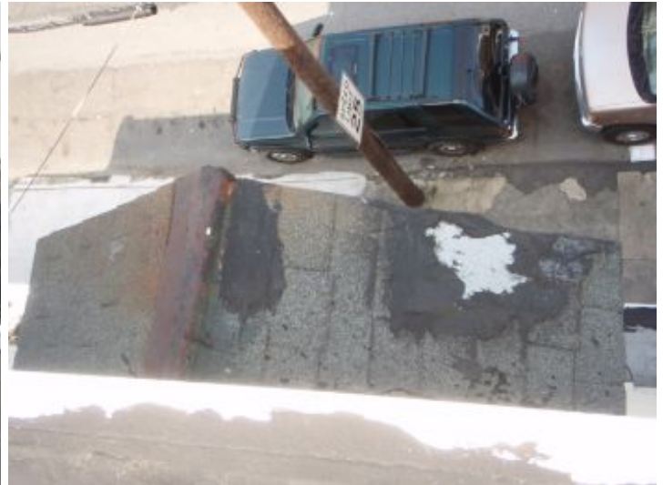
Damaged Dormer Window Roof
