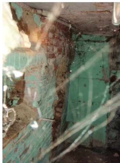
Foundation Wall Appears to be Bulging
