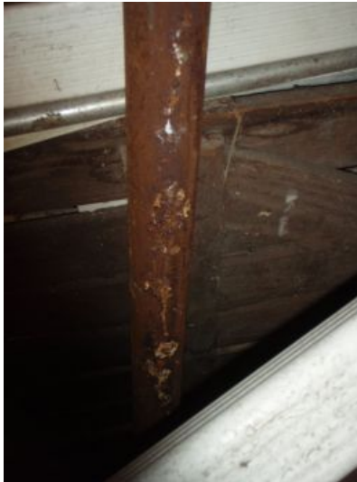
Cracked Cast Iron Waste Pipe in Basement
