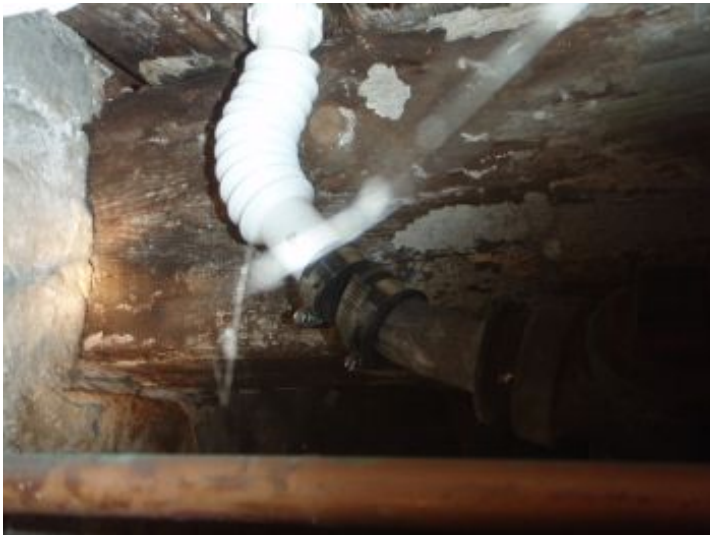
Improper Drainpiping in the Basement
