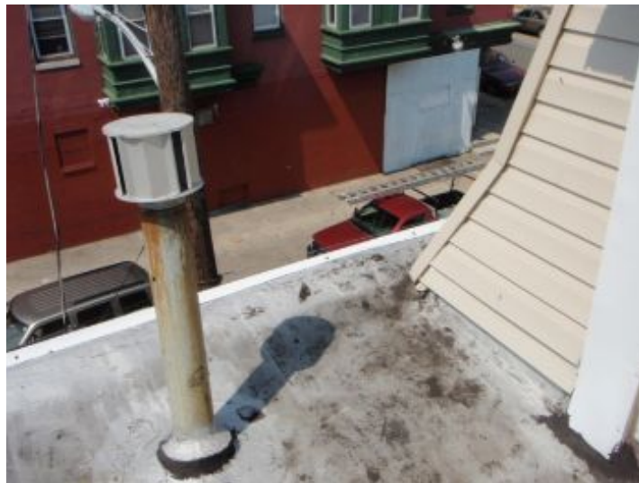
B-Vent for 2nd Floor Furnace is Too Close to the Exterior Wall
