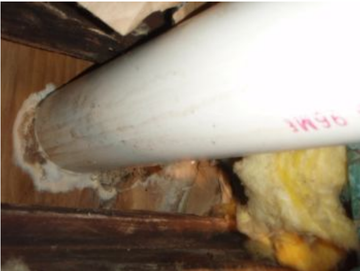
Rotting Subfloor Under Bathroom
