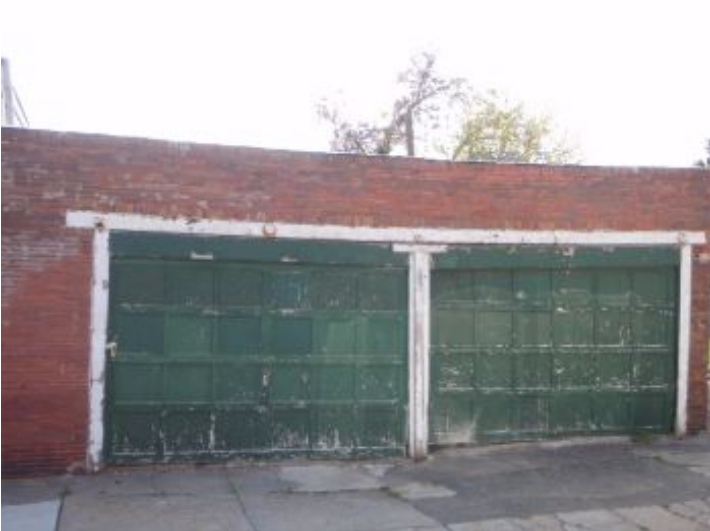
Sagging Door Lintel/Header
