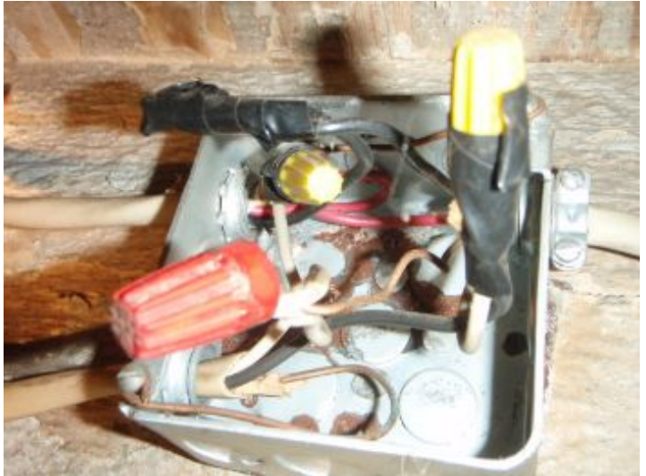
Ground and Neutral Wires Connected at Junction Box in Basement
