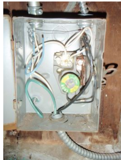
Overfused Circuit at Fire Alarm Panel
