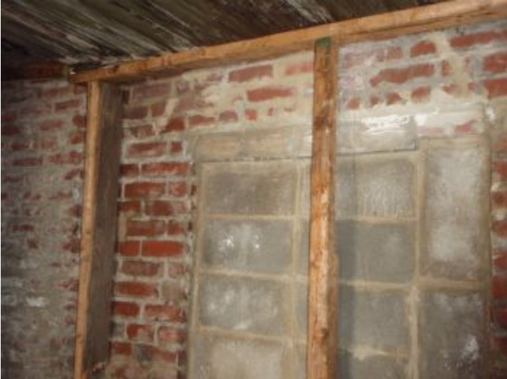
Rotting Roof Sheathing and Rafters
