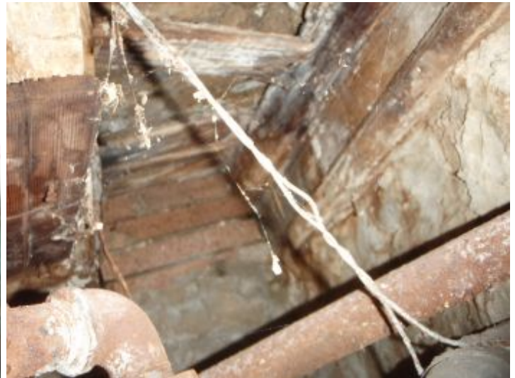
Rotting Flooring at Northwest Corner of Basement
