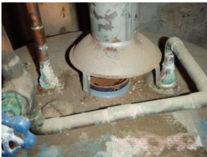
Draft Hood Improperly Installed
