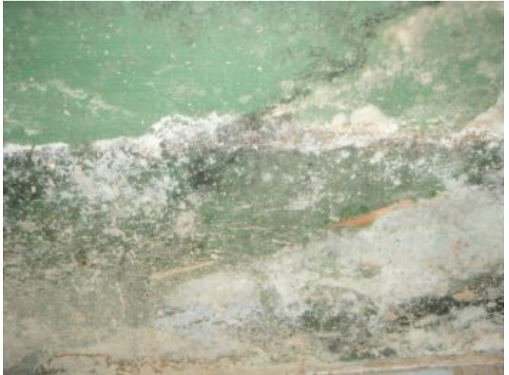
Possible Mold Staining on Finished Wall in Basement
