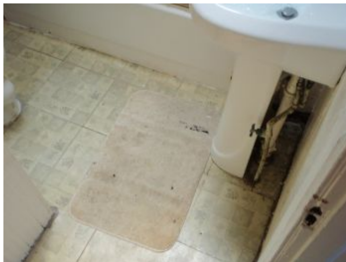
Moisture Damaged Flooring and Subflooring
