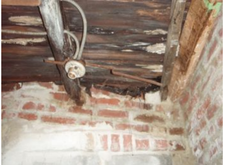
Rotting Roof Sheathing
