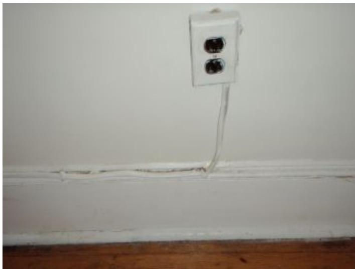
Exposed Wiring Run in 3rd Floor Bedroom
