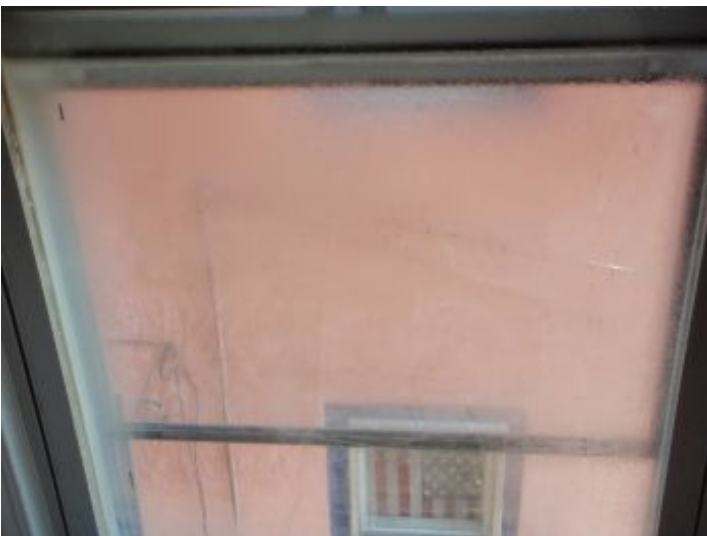
Failed Thermoseal at Window
