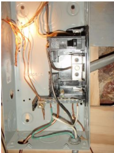
Improperly Wired Subpanel
