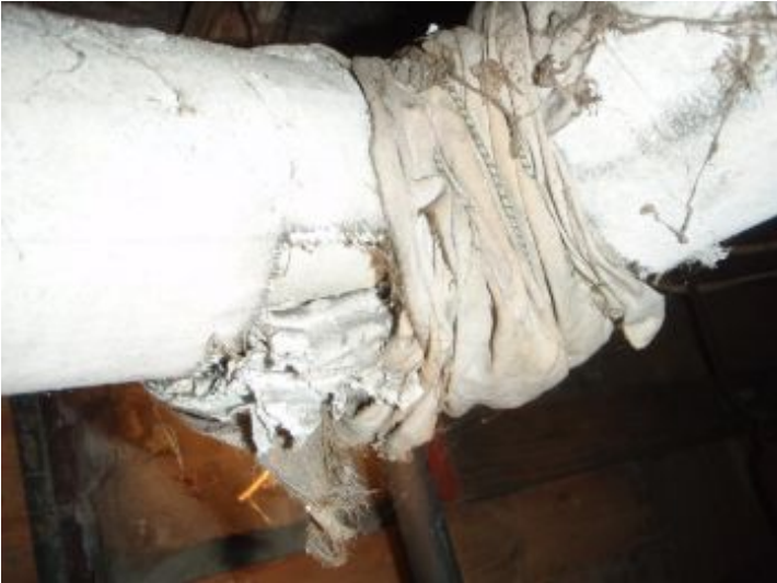
Possible Asbestos Containing Insulation in Basement
