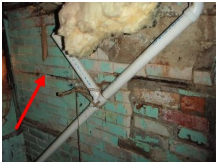
Horizontal Crack Noted in Rear Foundation Wall
