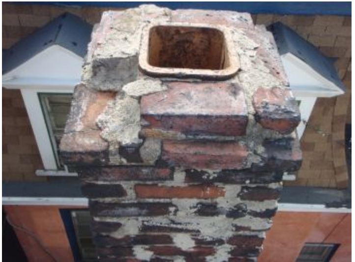
Chimney Crown is Deteriorating
