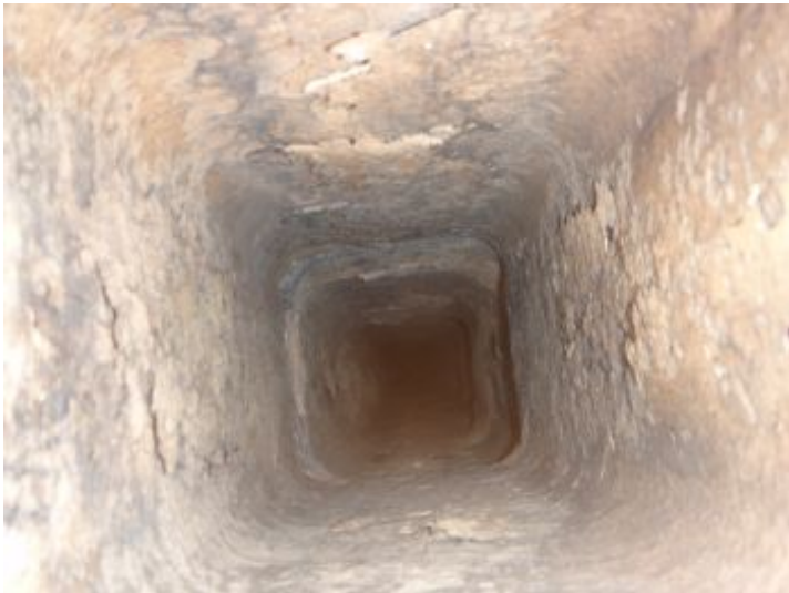
Deteriorating Chimney Liner
