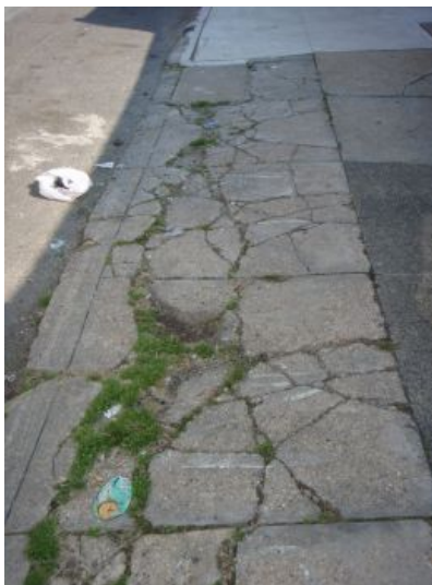
Major Damage Noted at the Driveway
