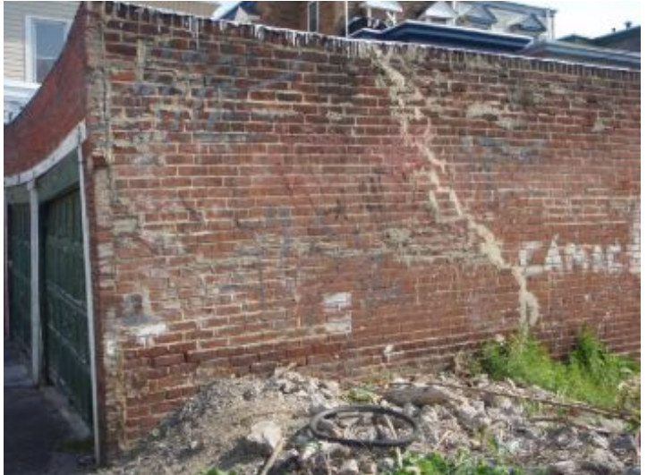
Signs of Major Structural Movement in the Garage Exterior Walls
