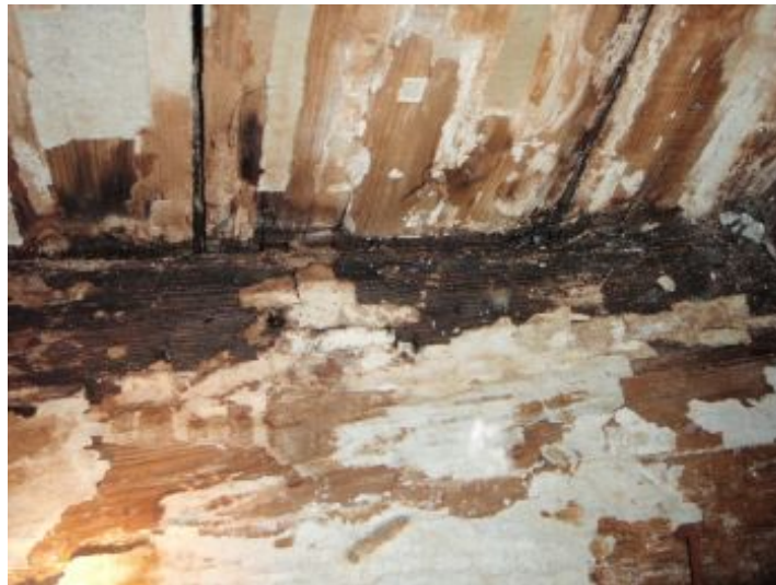
Rotting Flooring Under Bathroom
