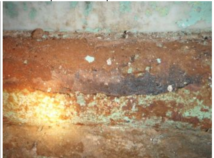
Cracked Cast Iron Waste Pipe
